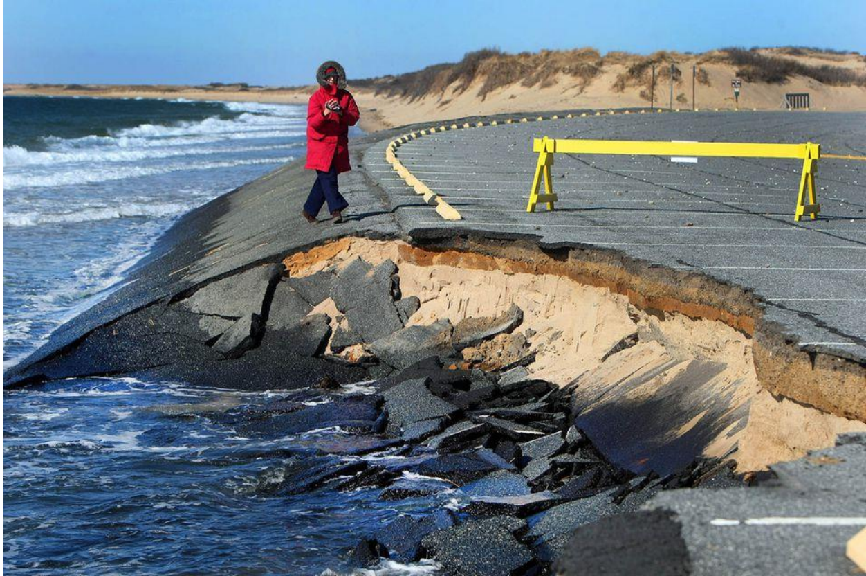
Erosion collapses a parking lot at Herring Cove Beach in Provincetown. JOHN TLUMACKI
