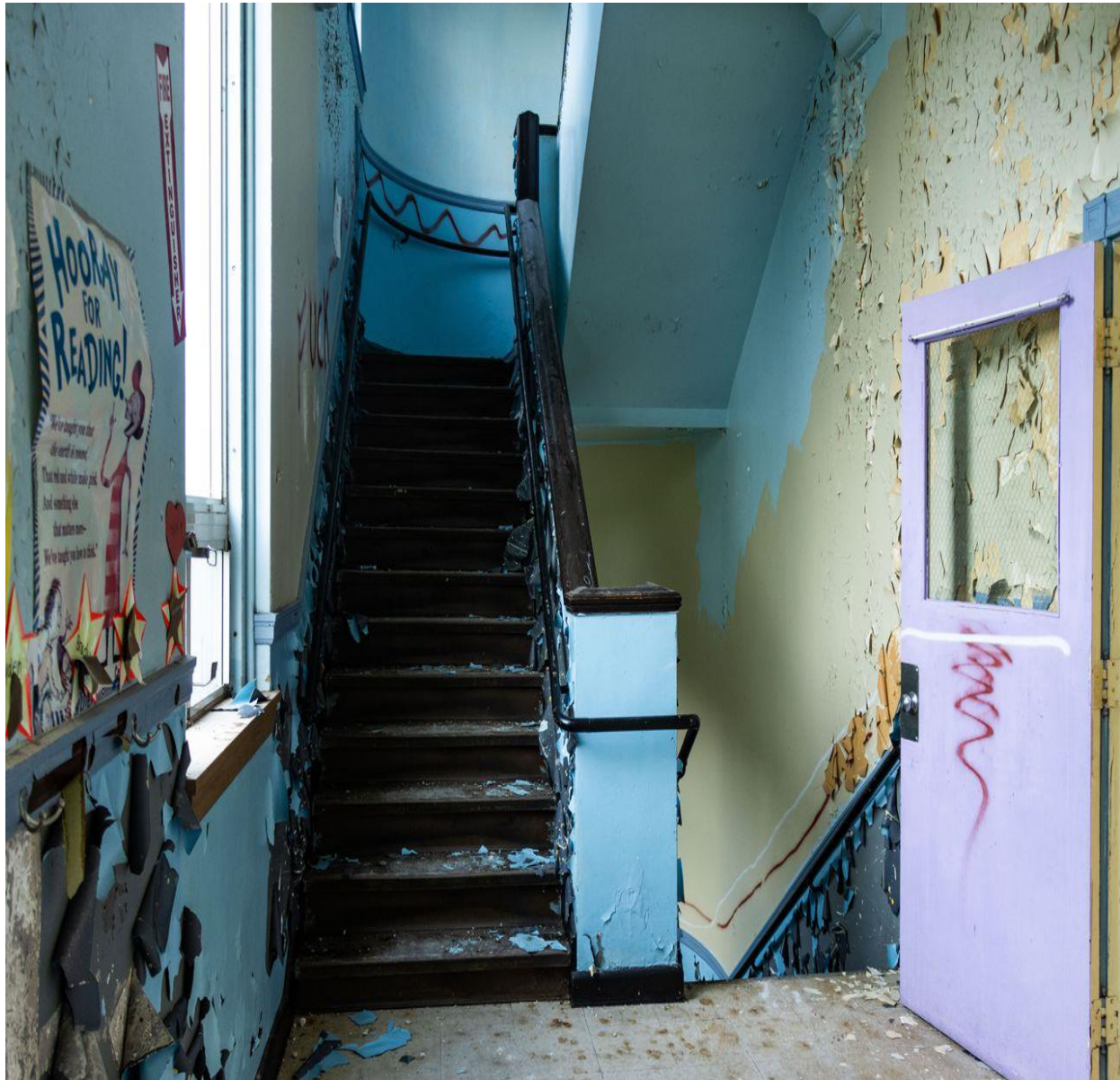
Inside the former Baldwinville School in Templeton, which will be redeveloped into apartments. (Tréa Lavery, MassLive)
