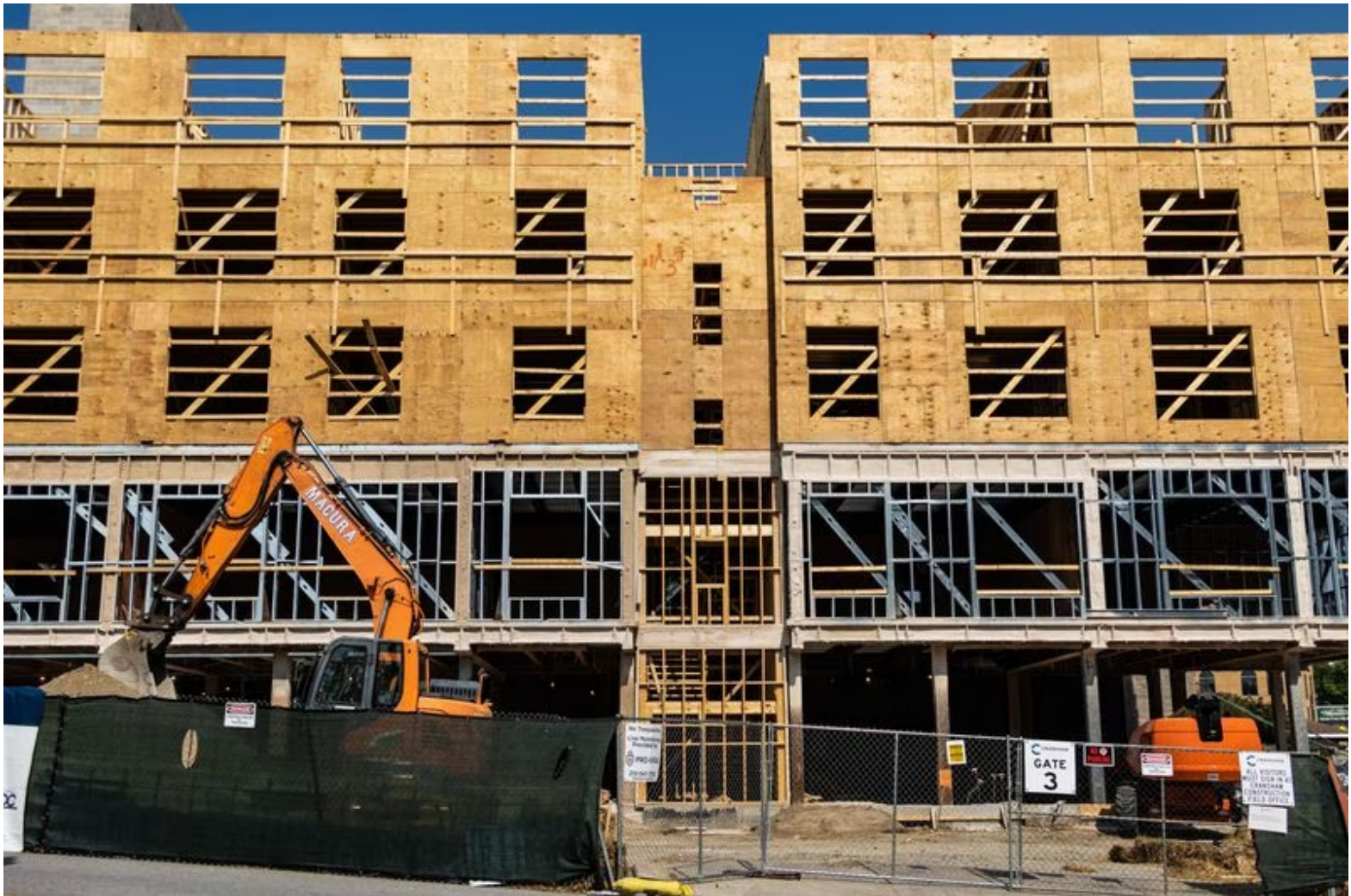
A six-story affordable housing development containing 83 apartments is under construction at the former Table Talk Pies property in Worcester. (Tréa Lavery, MassLive)
